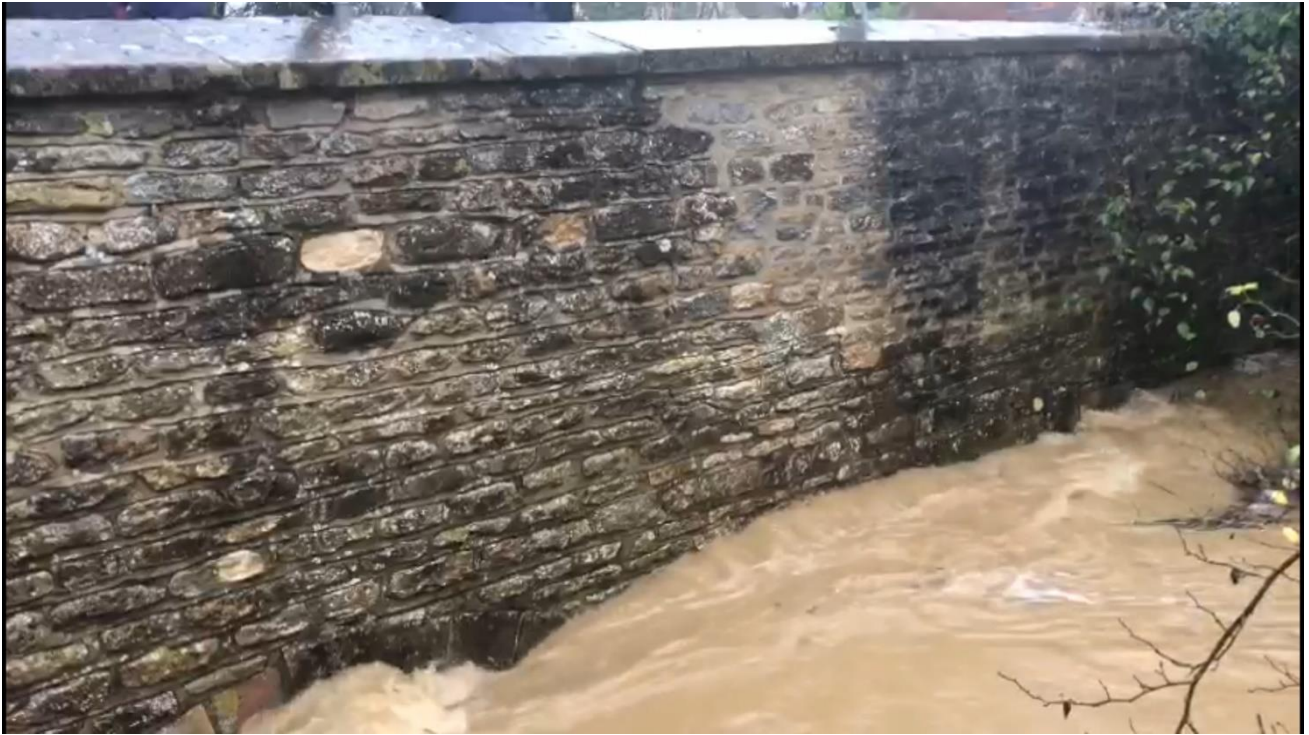
P17 Corston Road Bridge, Storm Bert
